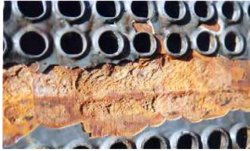
Fig. 2.9 Galvanic corrosion of coated carbon steel tube sheet because of high ratio between cathode (Admiralty brass tubes) and anode area (carbon steel tube sheet coated with epoxy). Gray – failed epoxy coating; yellow – rusted tube sheet. (For a full color version of this figure, see the Color Section)
