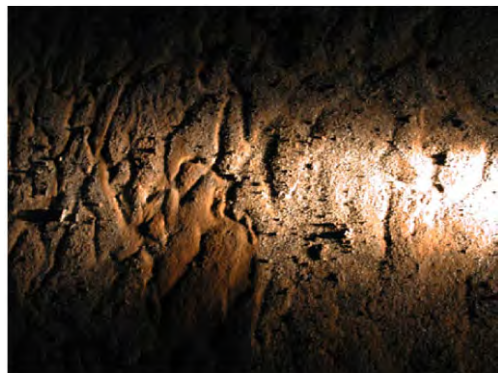
Fig. 3.17 Corroded bottom of a crude oil AST. The morphology of the surface and microbiological examination showed MIC. (For a full color version of this figure, see the Color Section)
