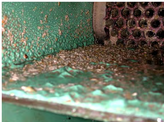
Fig. 3.2 Scale (calcium and magnesium carbonates) formed inside of heat exchanger with cooling water after 4 years. (For a full color version of this figure, see the Color Section)
