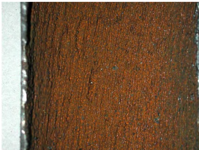
Fig. 2.16 Erosion-corrosion inside a liquefied petroleum gas (LPG) carbon steel tube. “Grooves” are formed as a result of erosion. (For a full color version of this figure, see the Color Section)
