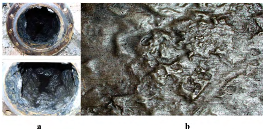
Fig. 2.14 (a) SRB inside cooling water carbon steel pipes (after four years); the thickness of biofilm with SRB was about 6 to 10 cm. (b) Corroded carbon steel bottom of the crude oil above-ground storage tank after 18 years of service as a result of SRB activity. (For a full color version of this figure, see the Color Section)
