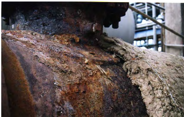
Fig. 3.9 Corrosion of a heat exchanger under thermal insulation. (For a full color version of this figure, see the Color Section)
