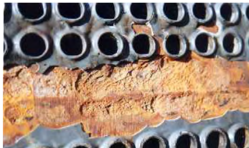
Fig. 2.9 Galvanic corrosion of coated carbon steel tube sheet because of high ratio between cathode (Admiralty brass tubes) and anode area (carbon steel tube sheet coated with epoxy). Gray – failed epoxy coating; yellow – rusted tube sheet.
