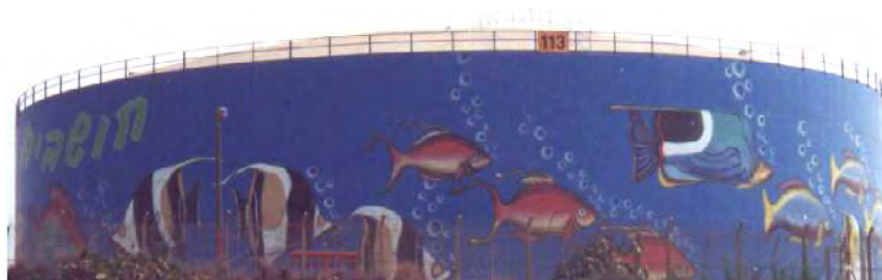
Fig. 6.15 Anti-corrosion protection as well as decoration of a storage tank (Israel). (For a full color version of this figure, see the Color Section)
