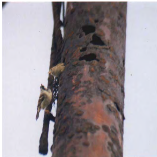
Fig. 6.24 “Corrosion led to contentment”. Corroded mast of a ship (Haifa Bay). (For a full color version of this figure, see the Color Section)
