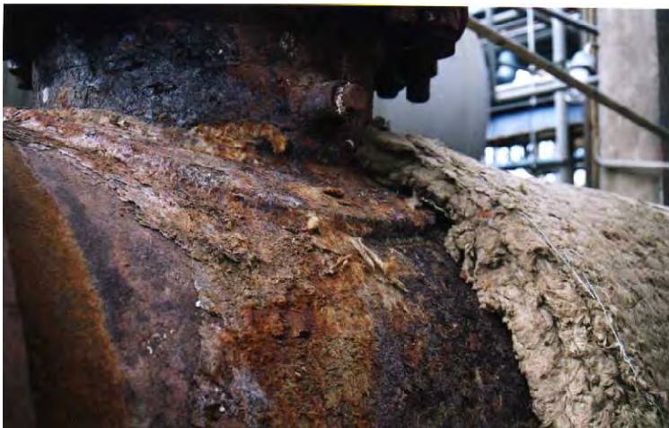
Fig. 3.9 Corrosion of a heat exchanger under thermal insulation.
