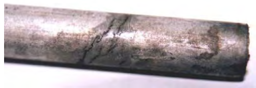
Fig. 2.17 Chloride stress corrosion cracking of an SS 316 tube in the atmosphere containing HCl gas.
