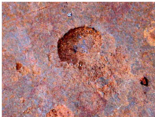
Fig. 2.10 MIC on a metal surface compared with pitting, crevice, differential aeration cell, or galvanic corrosion. The bottom of a crude oil storage tank after a microbial attack. (For a full color version of this figure, see the Color Section)
