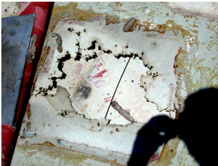
Fig. 3.15 Corroded roof of the gas oil AST after 5 years of service.
