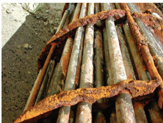
Fig. 2.6 Heat exchanger: tubes made of titanium and baffles made of carbon steel (cooling water, 4 years). Deposits on the titanium tubes are the salts (scale) formed from the cooling water, and not corrosion products. (For a full color version of this figure, see the Color Section)
