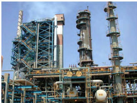
Fig. 3.3 Metallic structures and equipment in the atmosphere. (For a full color version of this figure, see the Color Section)
