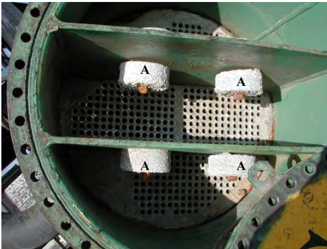
Fig. 4.8 Aluminum sacrificial anodes (A) installed on the inside of heat exchangers coated with epoxy paint (green). The cooling water flows inside the tubes.
