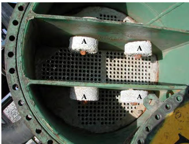
Fig. 4.8 Aluminum sacrificial anodes (A) installed on the inside of heat exchangers coated with epoxy paint (green). The cooling water flows inside the tubes. (For a full color version of this figure, see the Color Section)
