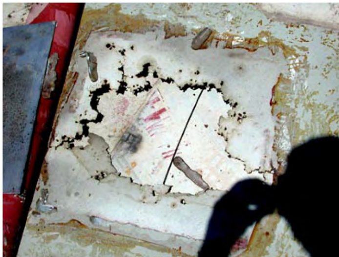
Fig. 3.15 Corroded roof of the gas oil AST after 5 years of service. (For a full color version of this figure, see the Color Section)
